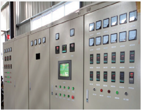
Electrical control system
